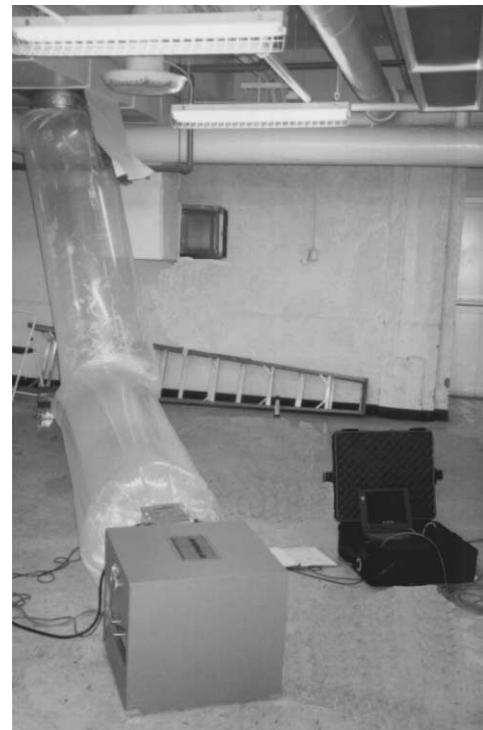
Fig. 4. Aerosol injection machine connected to Building LS-2 via 0.65 m (25.5 in.) diameter lay-flat polyethylene tubing.
