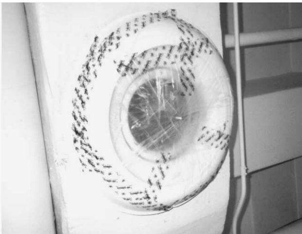
Fig. 3. Sealed diffuser in Building LS-2.
